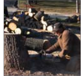
Contractor cuts big stump to make room for remodeling the first tee.
